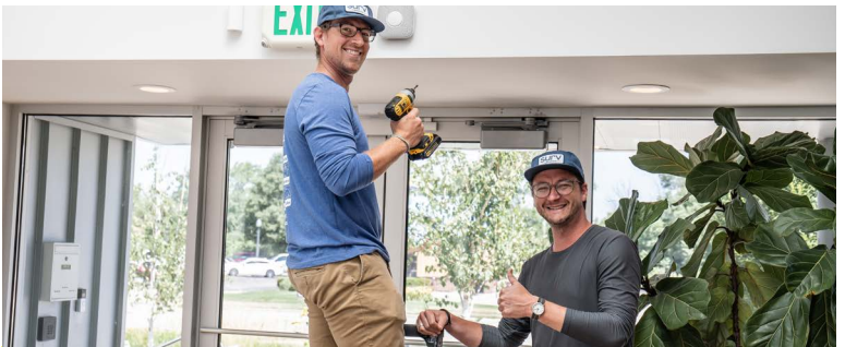
Our friends at Surv Lakeshore stopped by to install brand new smoke detectors throughout our office.
